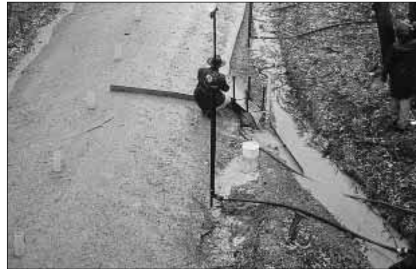
Well-used, unsealed road in the Cuttagee Creek catchment showing runoff entering a mitre drain, used to divert runoff onto the adjacent hillslope
