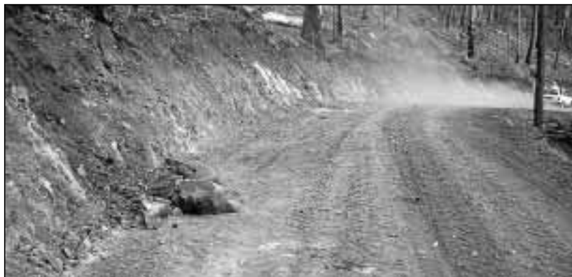
Feeder access road cut into hillslope in Cuttagee Creek - the road is drained by outfall drainage i.e. all water is diverted to the fill-side of the road by sloping the road outward
