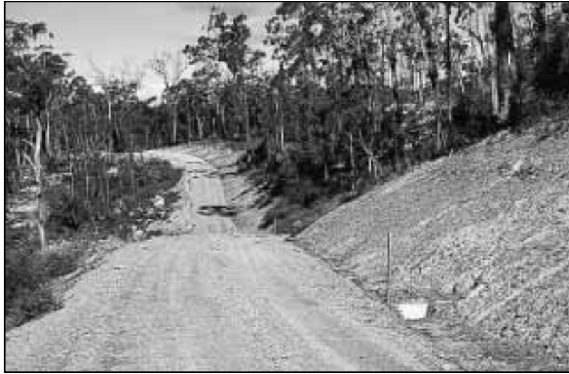
A cut-and-fill road showing cut-batter used to drain a segment of road in a mid-valley position where mitre drains cannot be installed
